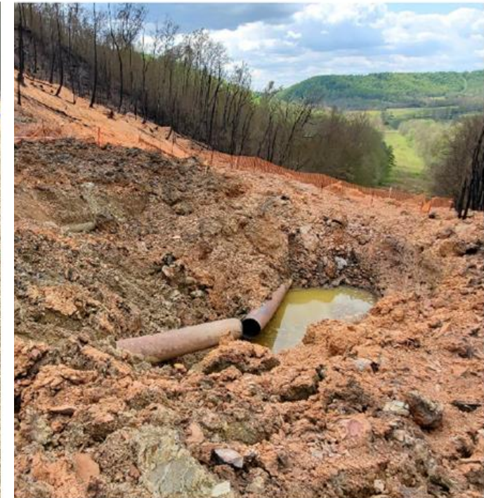
Figure 1. Ruptured pipeline. Source: BGC Engineering USA, Inc.)
